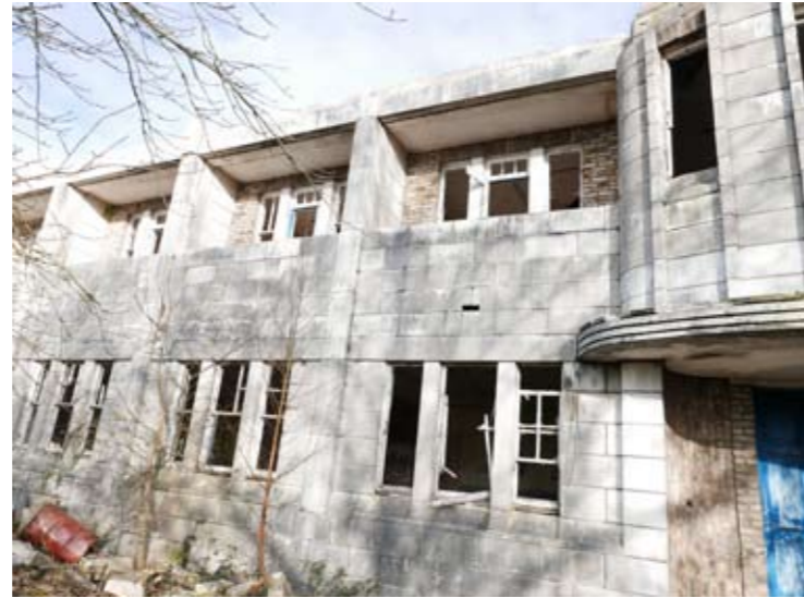
Picture 33: Building 9. The South elevation of the former Officer's Mess. It has deteriorated significantly and many of the openings having been badly damaged or destroyed
